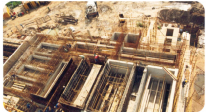
Figure 1 Construction of the Durban Wastewater Recycling Plant (Photo credit: Ethekeweni Metro Water Services)
